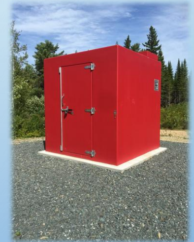
Eel Ground, NB - Well head protection by enclosure.
